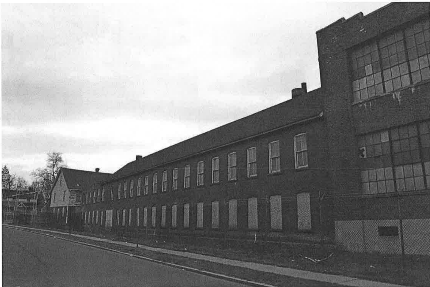
West (side) elevation of factory showing c.1900 and 1903 additions from Love Lane. Camera facing northeast. Photograph 4 of 18.
