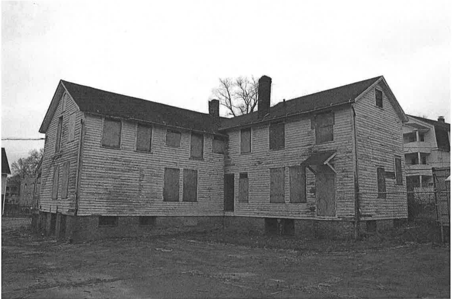
North (rear) and east (side) elevations of Swift homestead (c. 1887) from interior of property. Camera facing southwest. Photograph 12 of 18.
